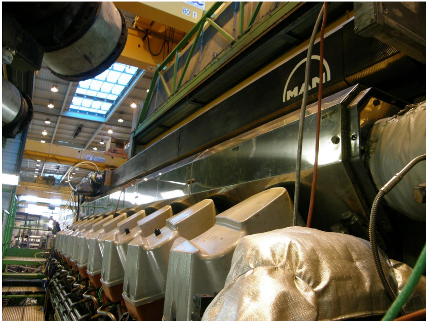
The 20V28/33D prototype engine on the test bed in St. Nazaire
