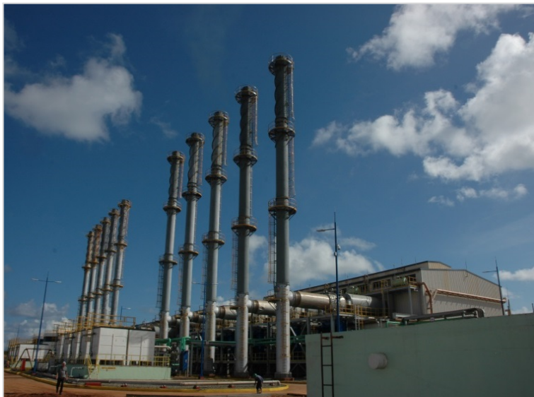
184 MW Power Plant in Moa, Cuba
